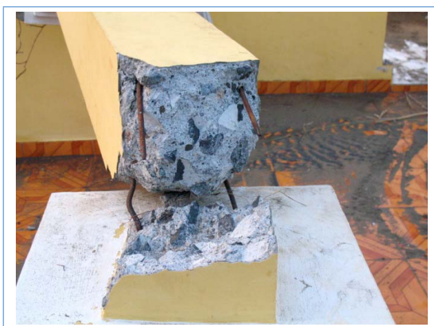
Figure 1 Column component after collapsing during the aftershock
