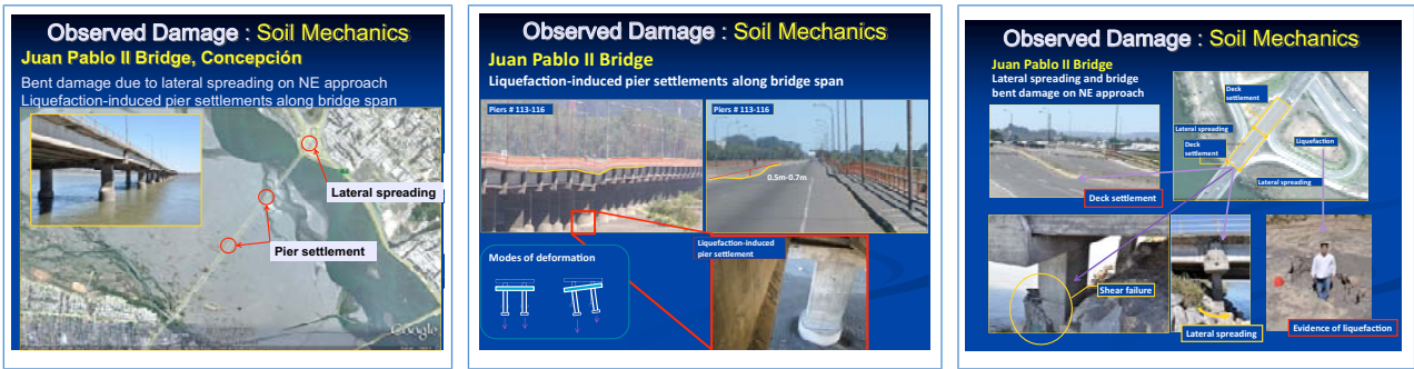
Figure 19 Bridge failure due to liquefaction and settling
