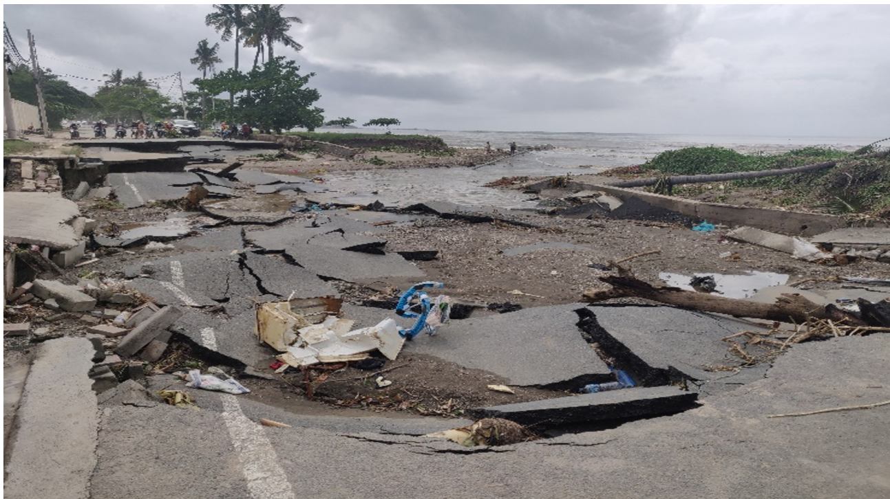
Photo 2: Damage Caused by Flooding in the Capital of Dili in April 2021
