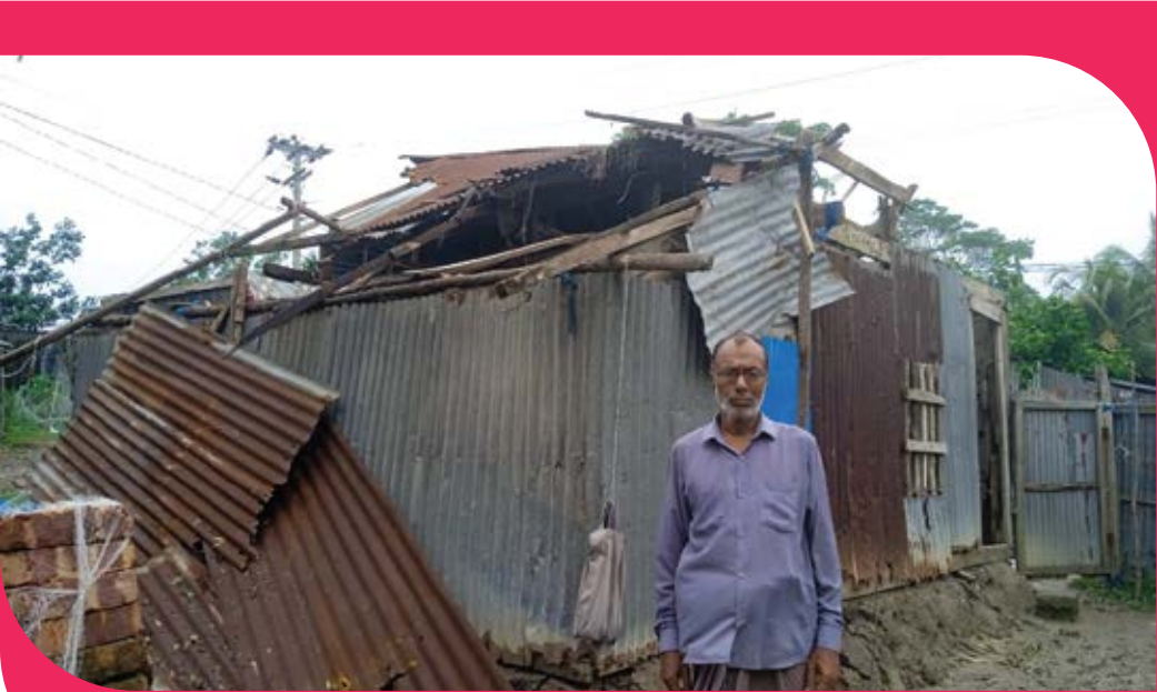
Photo: Wind Gust from Cyclone Remal tore off the tin roof, leaving the house damaged (Credit: STEP Consortium).
