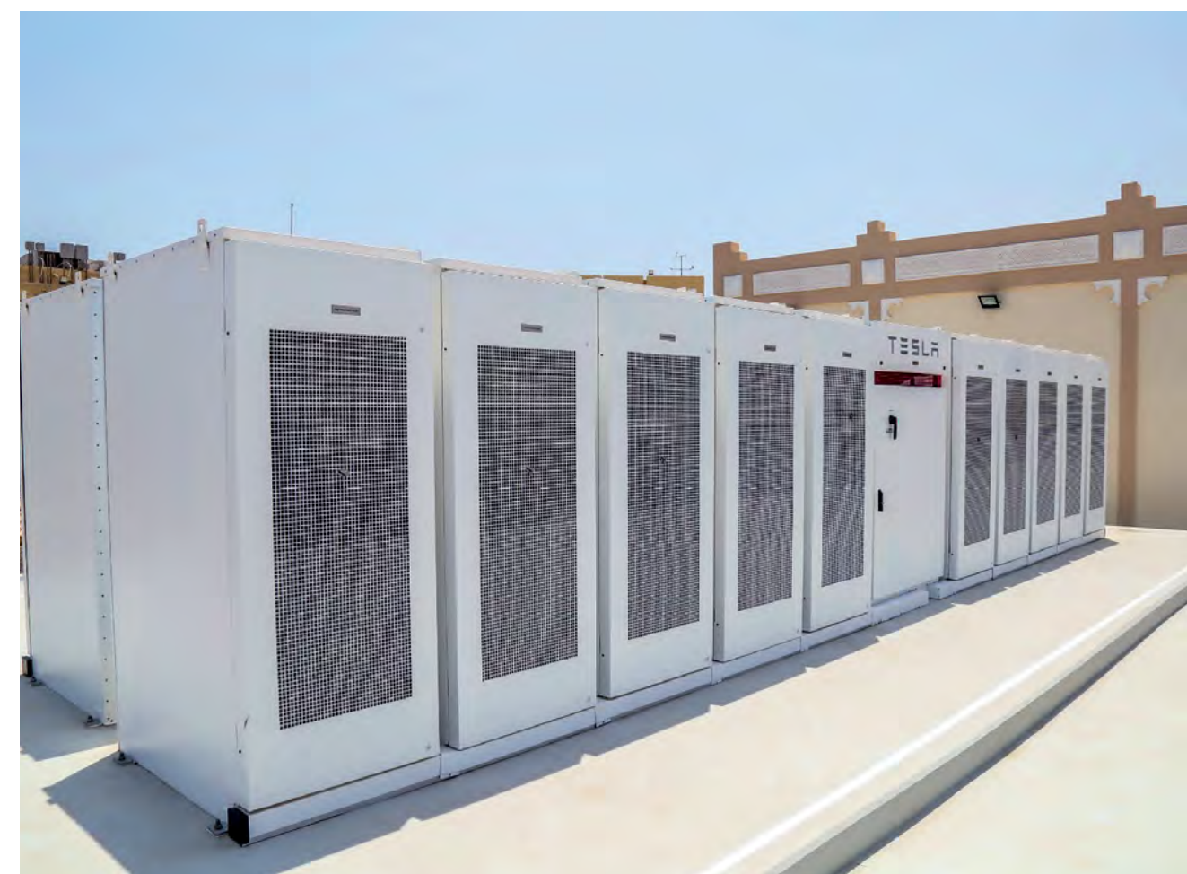
Kahramaa Battery storage power station.
